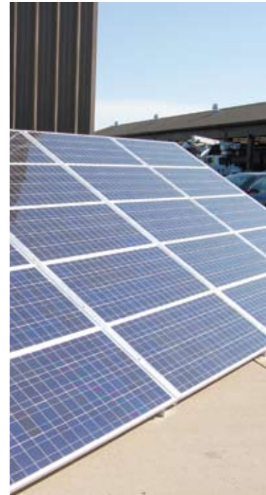
Solar-panel array at Butler Rural Electric Cooperative near Oxford, Ohio.
