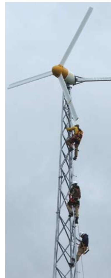
Buckeye Power and Logan County Electric Cooperative installed a demonstration 10-kilowatt wind turbine at Indian Lake High School in 2006.
